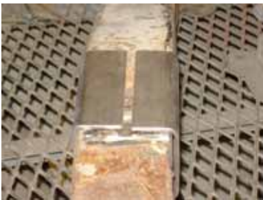
THIS PHOTO SHOWS THE SIDE VIEW OF THE RAIL WITH THE CHANNELS IN PLACE
